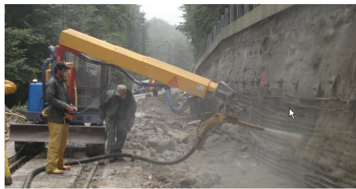
Picture on the left: Mounting of the AL-302 onto a Putzmeister carrier
